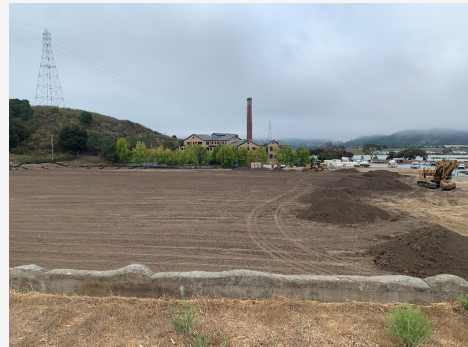
Topsoil being installed over the cleanup area at Larkspur Landing on August 25. Remaining work involves planting vegetation by hydroseeding.
