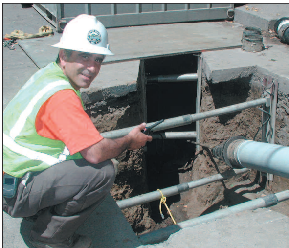
Assistant Engineer Dennis Gavallos monitors the bursting head and new pipe as the process begins.
