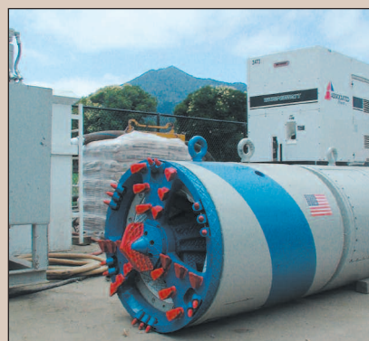
The business end of the 22-foot laser-guided drill used in the project.
